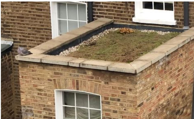
Sedum roof on a rear extension in our area helping to address climate change.
