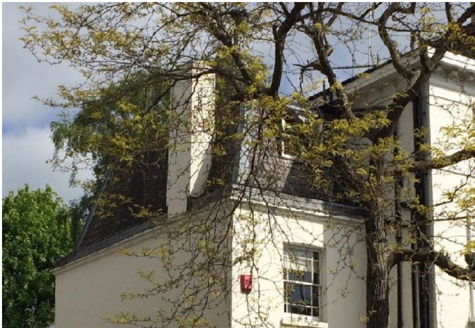
This roof outside of our area shows the chimney raised and incorporated into the sloping roof pitch. End of terrace hipped roof mansards on Needham Road showing their greater useful internal volume for passive cooling and energy saving equipment. Using slate or tiles consistently on all pitches contributes to visual uniformity and ease of construction and detailing.
